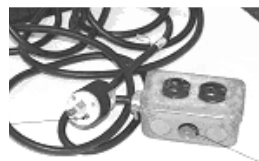
Box with missing knockout and missing ground pin must not be used.
