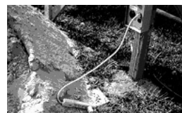
Improper use of power strip—not intended for outdoor use (wet or damp locations—don't use it!)
